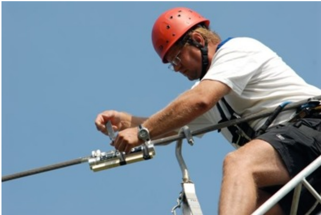
Pict. by courtesy of BEWAG Netz GmbH
