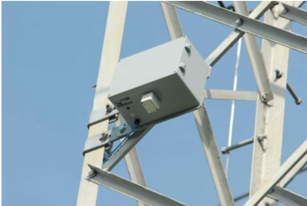
Pict. by courtesy of BEWAG Netz GmbH
